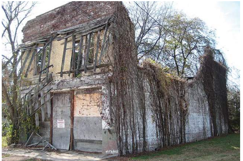
The decaying grocery store in Money where the Emmett Till story is rooted is one of the MDNHA’s most significant resources in need of urgent help.
